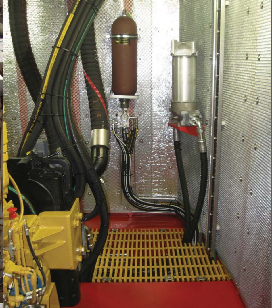
Seatrac: Fully Enclosed Machinery Room
